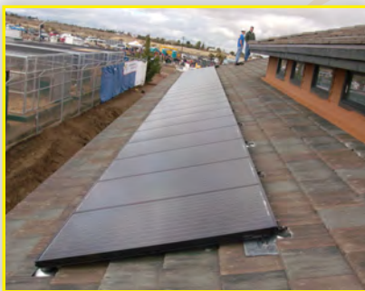
24 Andalay 175 watt Modules, 1 Fronius 4000 Inverter- (4.2 kW) installed Feb 2009
